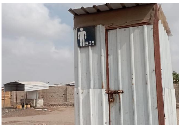
Emergency Latrines for Male Installed in Al-Ribat IDP Camp as Part of WASH Response May, 2025
