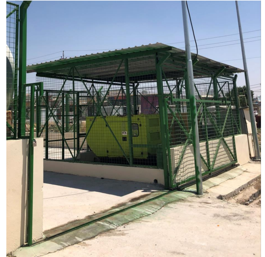
Reorganized generator station and electricity plant at Domiz 2 camp.
