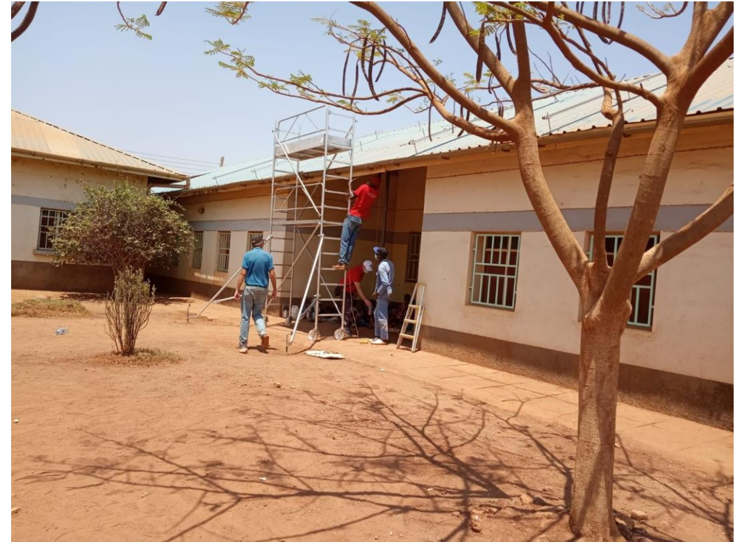
Maintenance of the solar panels of the Hospital with the expatriate technician
